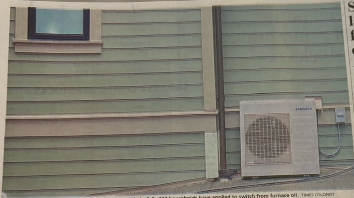
A heat pump at a house under construction in Saanich. In B.C., 327 households have applied to switch from furnace oil. TIMES COLONIST
